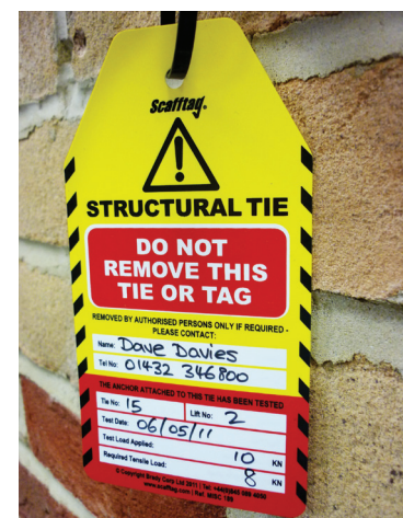
Legend: Do Not Remove Scaffold Tie
