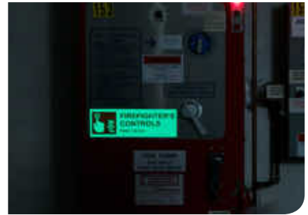
Exit & directional signs
