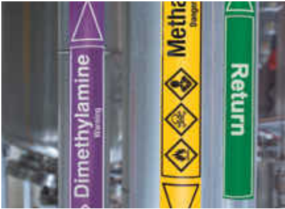
Pipe & valve marking
